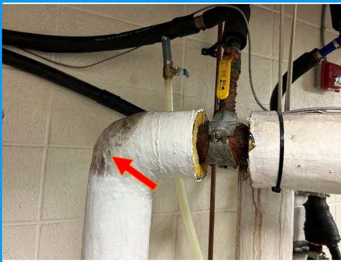
Photo 1: View of visible suspect mould growth (see arrow) on an asbestos containing parging cement insulated pipe fitting in the penthouse mechanical room of the subject building.
