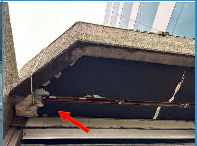
Photo 6: View of the asbestos containing Transite cladding (see arrow) observed on the soffit above the garage loading dock.
