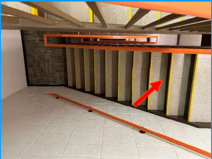
Photo 4: Typical view of asbestos containing 12"x12" tan with brown and white streaks vinyl floor tiles (see arrow) observed on stair treads in stairwells of the subject building.
