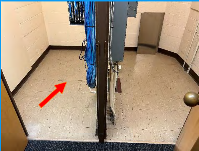
Photo 3: Typical view of asbestos containing 12"x12" tan with brown and white streaks vinyl floor tiles (see arrow) observed in the electrical equipment rooms of the subject building.
