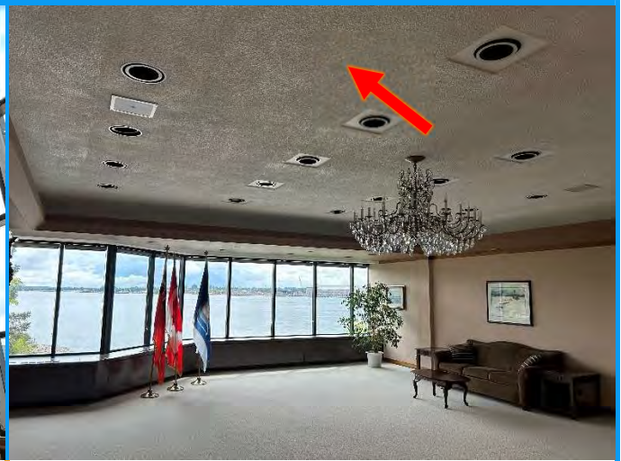
Photo 8: View of the asbestos containing textured finishes (see arrow) observed on the ceiling in the 3 rd Floor Hamilton Room.
